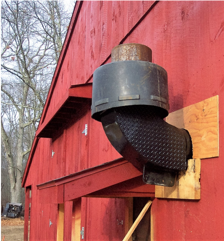
The exhaust for the Fairbanks Morse engine fabricated by Ed Bezanson.
